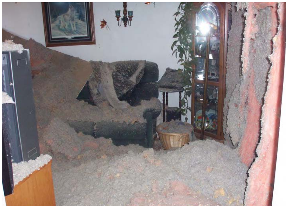
The aftermath in Laura's front room after the ceiling collapsed, covering everything with mountains of fiberglass insulation from the attic
